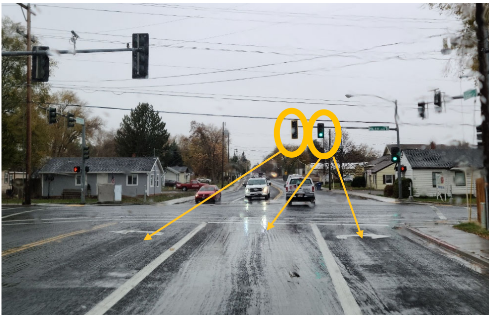
FIGURE 19: INTERSECTION SKEW AND MISALIGNMENT OF SOUTHBOUND SIGNAL HEADS
