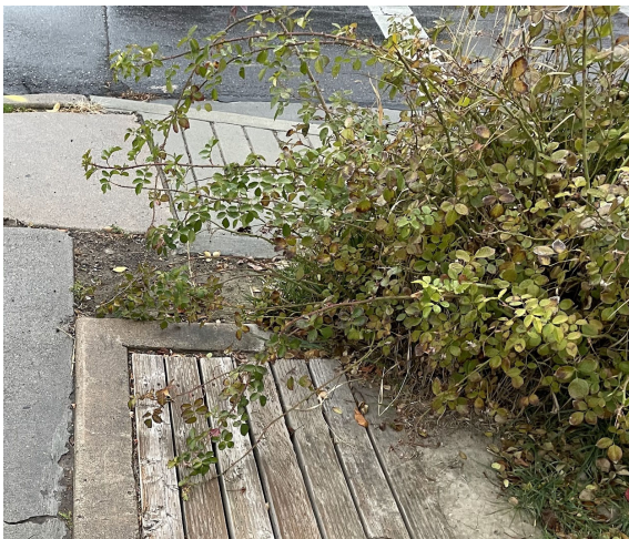
FIGURE 10: VEGETATION GROWTH CAN BLOCK DRIVER VIEW
