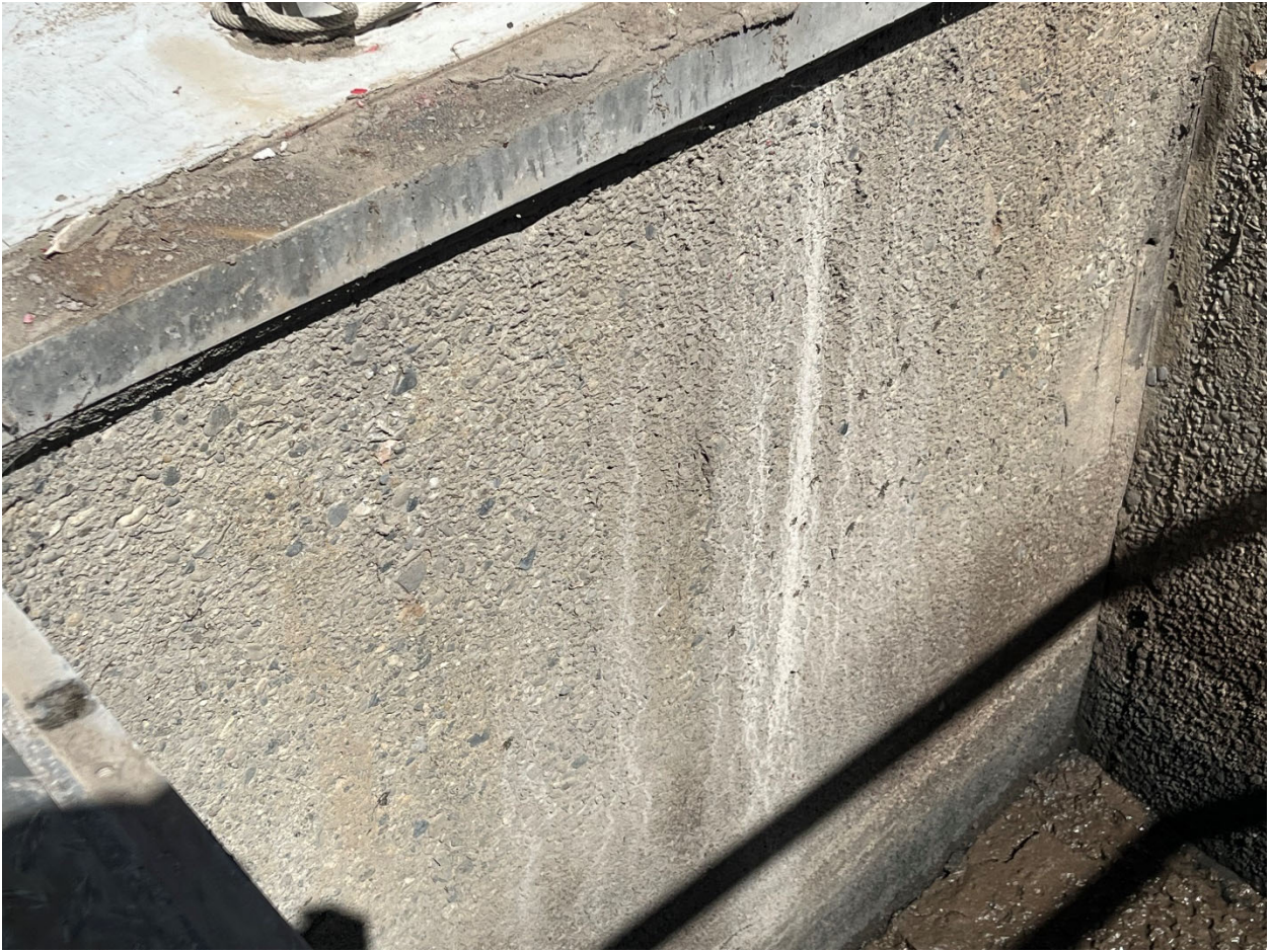
Photo 22: Paste loss and exposed aggregate in digester overflow box
