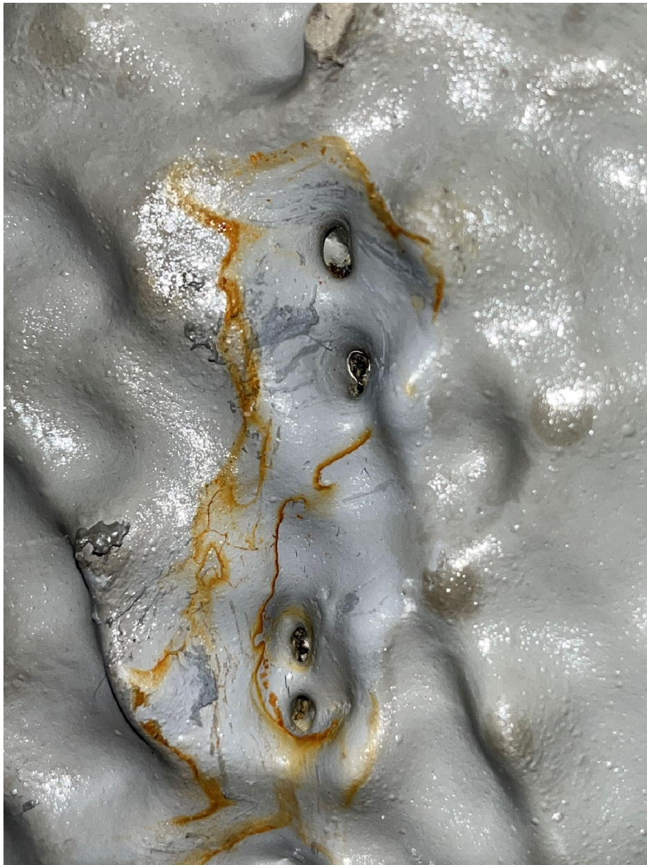
Photo 10: Pinhole in coating on digester cover interior with easily removed pinhole repair material, showing bare concrete below
