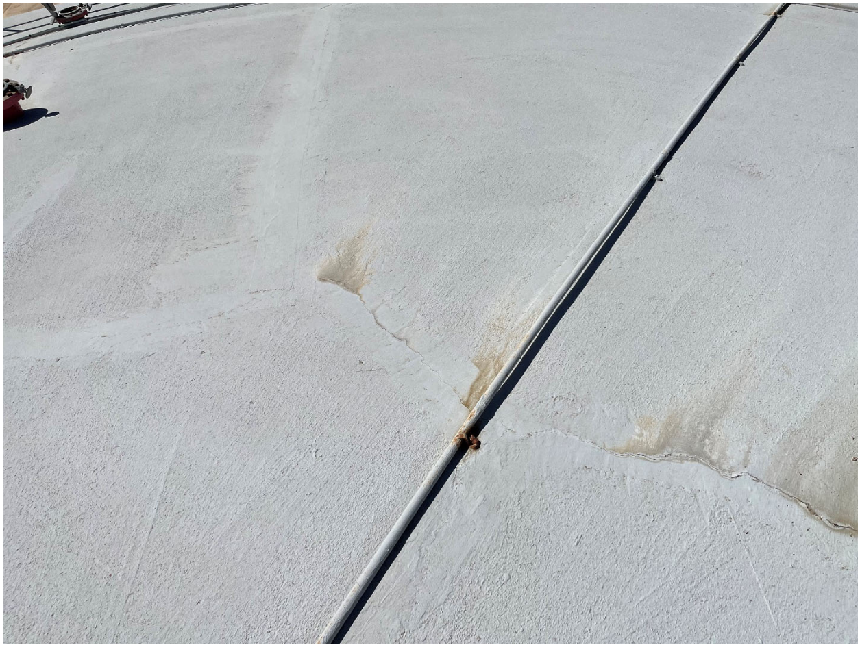
Photo 19: Multiple shades of grey coating present on digester cover exterior
