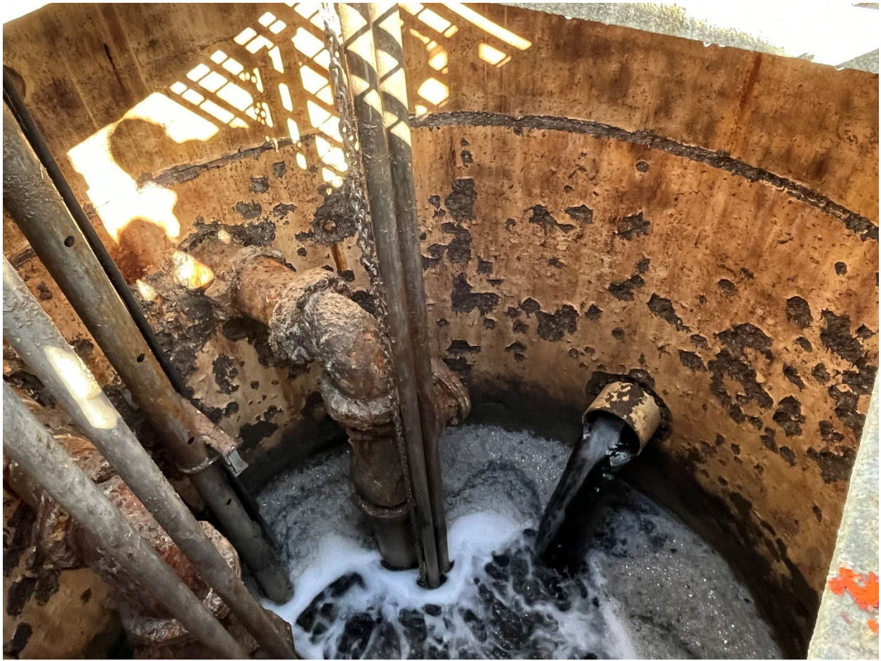
Photo 24: Overall view of filtrate pump station
