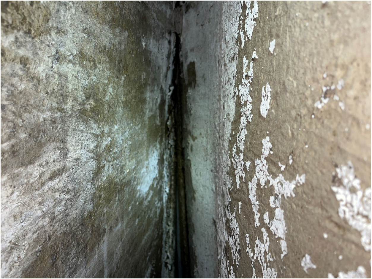
Photo 4: Between topcoat (right) failure and well adhered prime coat (left) on digester skirt interior (prior to existing coating removal project)
