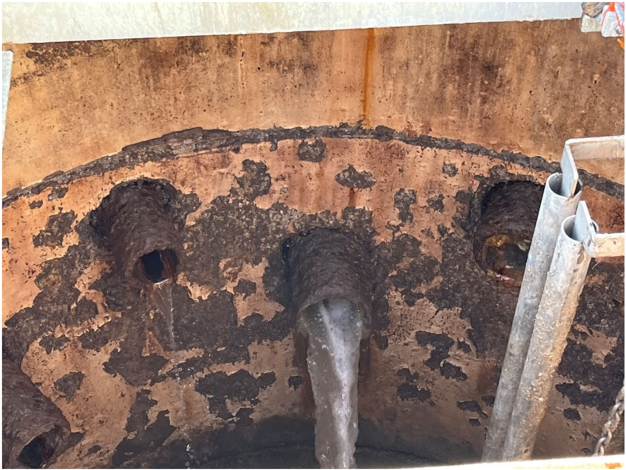
Photo 25: Pipe penetrations with increased cement paste loss at filtrate pump station
