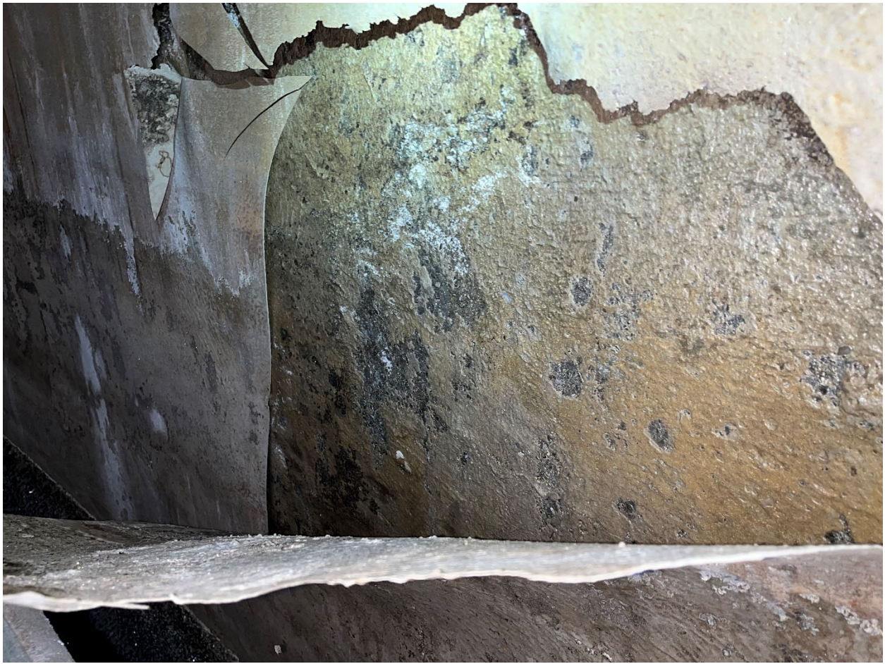
Photo 3: Topcoat failure and spot prime coat failure exposing underlying concrete on digester skirt interior (prior to existing coating removal project)
