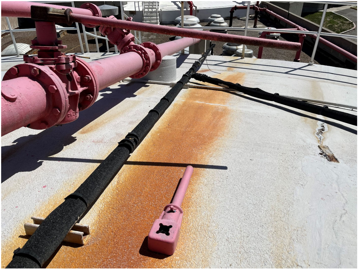
Photo 14: Staining on digester cover exterior and coating failure near cracking in digester cover exterior
