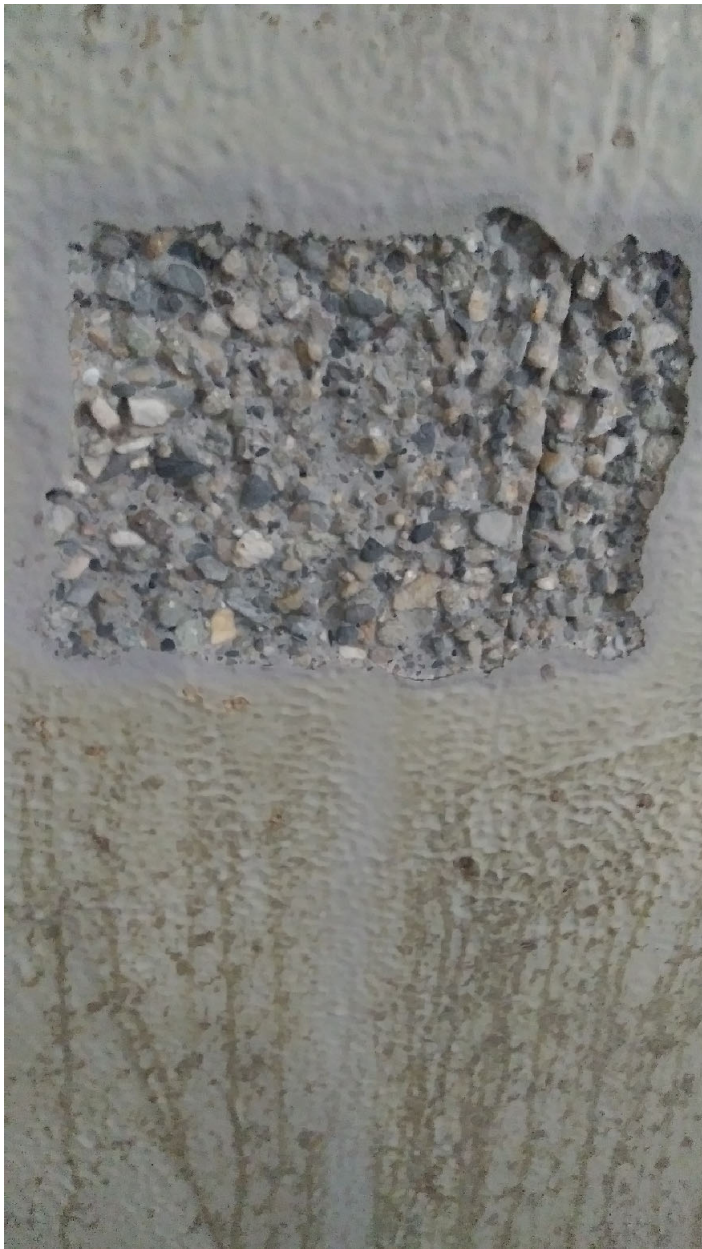
Photo 27: Coating removal at interior lid (Note exposed concrete aggregate due to over blasting). Concrete is assumed to be in good condition under the well-adhered interior dome coating
