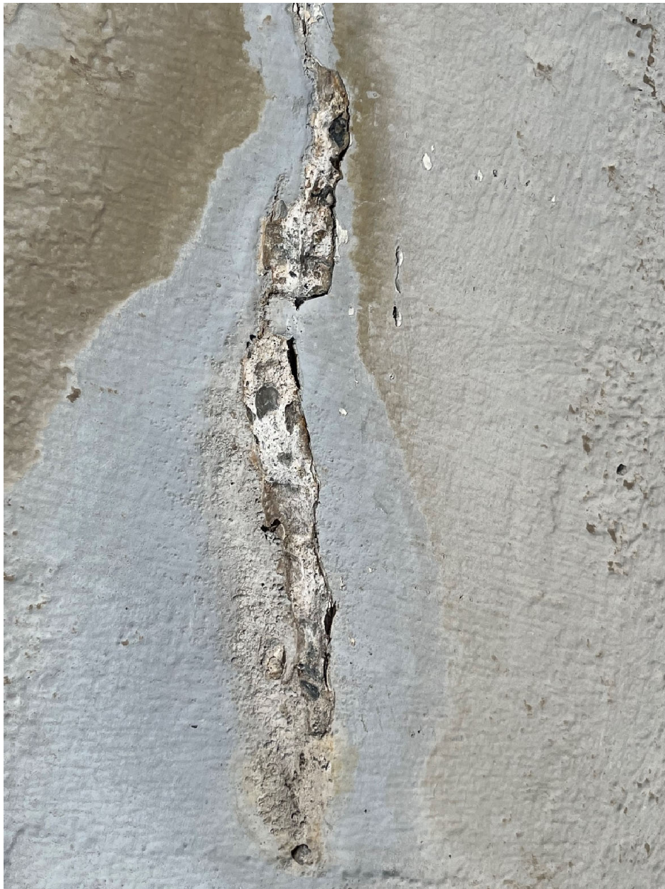
Photo 18: Close view of coating failure near cracking in digester cover exterior
