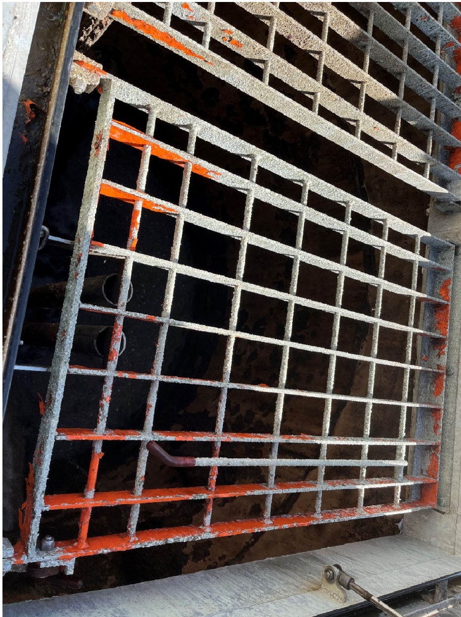
Photo 23: Grating coating failures and corrosion at filtrate pump station
