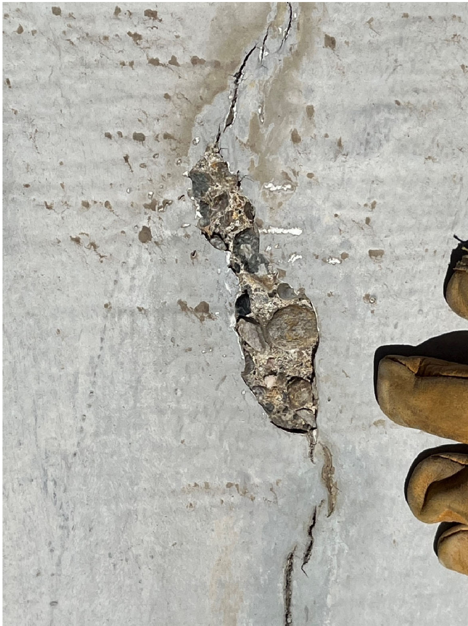
Photo 17: Close view of coating failure near cracking in digester cover exterior
