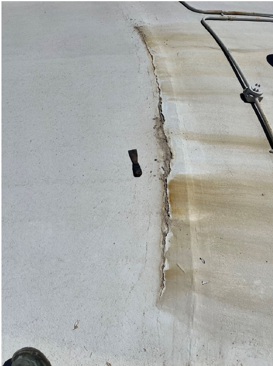
Photo 15: Coating failure near cracking in digester cover exterior
