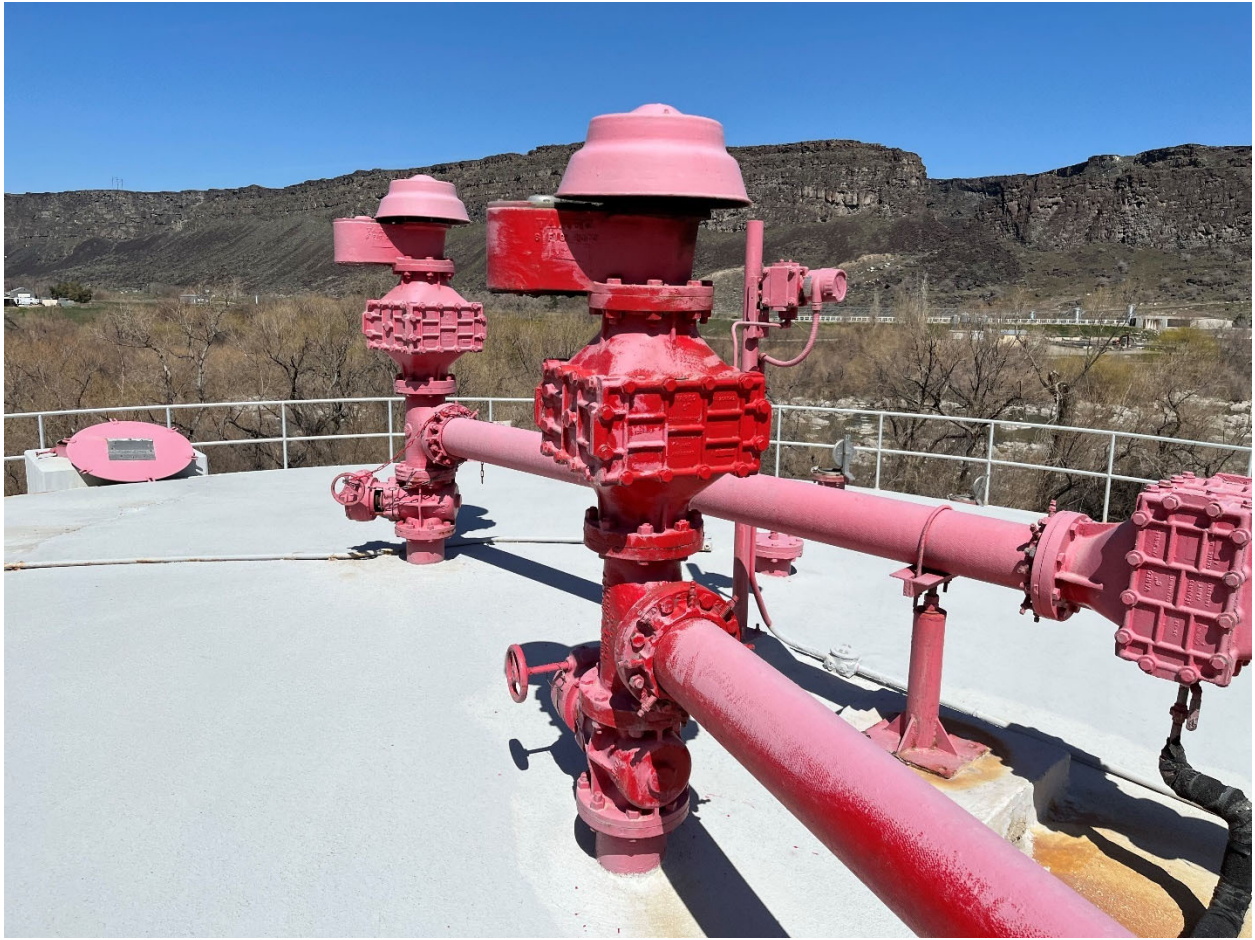
Photo 20: Aged pipe coatings are faded, and repair coatings are not well blended
