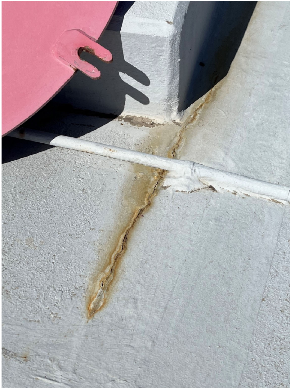
Photo 16: Coating failure near cracking in digester cover exterior
