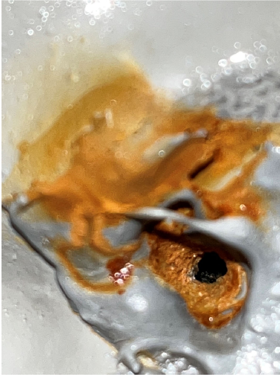
Photo 11: Close view of pinhole on digester cover interior with pinhole repair material removed, showing staining and concrete below
