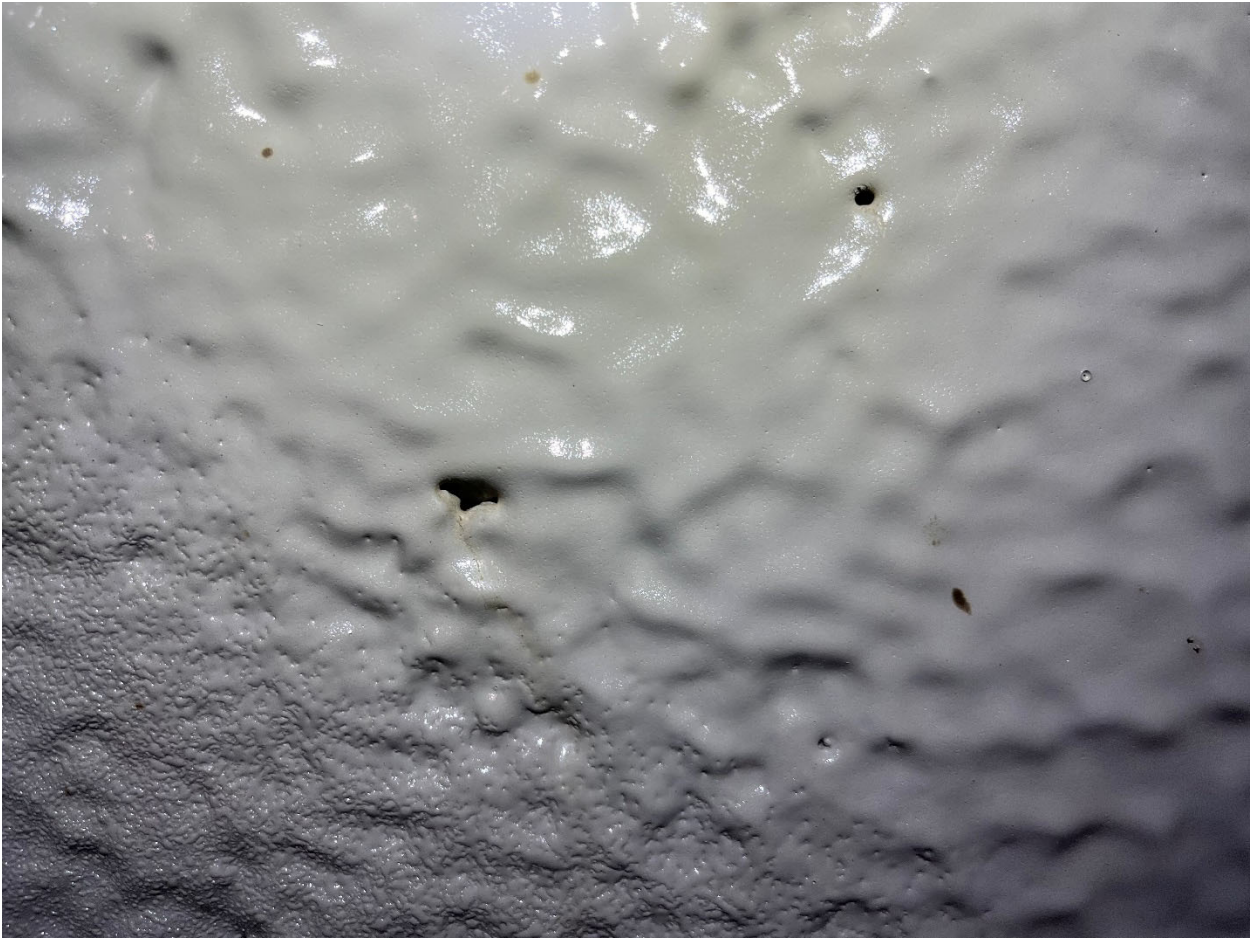
Photo 9: Pinholes in coating on digester cover interior
