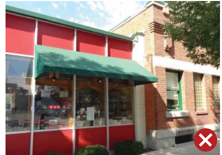
Inappropriate material selection.
