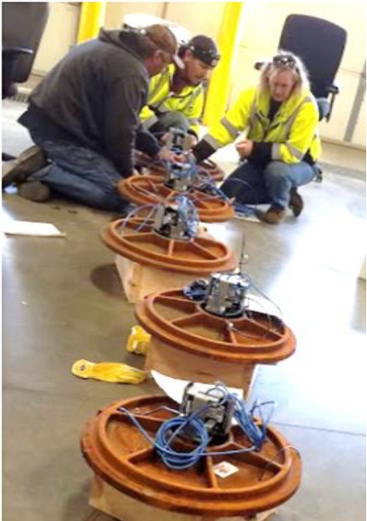
Aurora staff check and prepare to relocate SmartCover units without confined space entry
