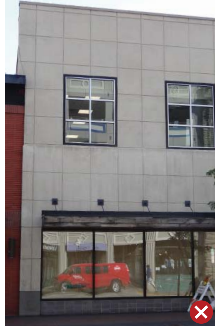
Inappropriate material selection.
