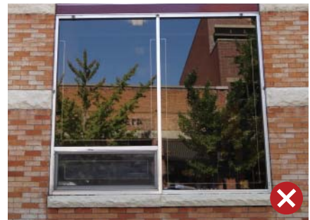
Inappropriate window replacement style.
