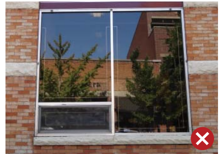
Inappropriate window replacement style.
