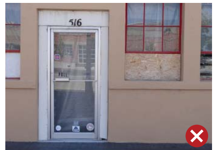
Inappropriate material and scale for opening.
