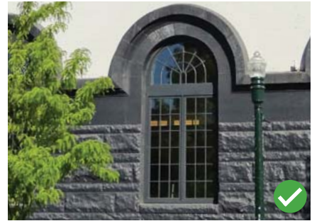
Appropriate historic window replacement.
