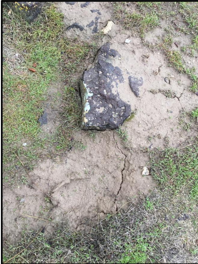
Photograph 5. Site conditions, looking at 1/4 inch tension crack , north of the project site, between side walk and canyon rim.
