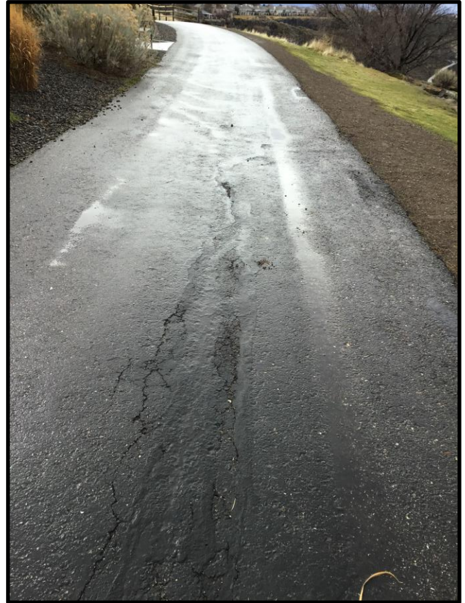
Photograph 10. Site conditions, looking north along paved walking path north of Twin Falls Visitor Center. Arcuate cracking ¼-inch wide and running parallel to canyon rim observed on path, possible evidence of ground settlement.
