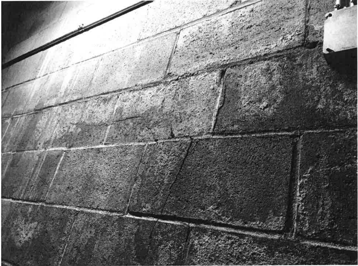
Spalling masonry on bearing wall below mezzanine floor
