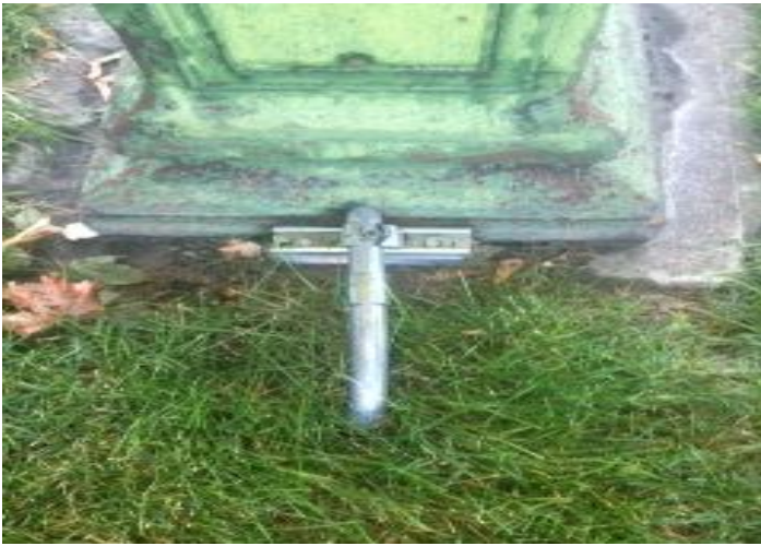
Figure 3. Light on 147 Lincoln Street. To restore power, the homeowner drilled conduit directly into the base of the streetlight, compromising the structural integrity of the cast iron.
