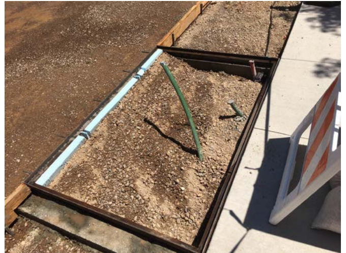
Block 1 – Shoshone to Gooding, Tree Well location with irrigation and power for decorative lighting, 28JUN2017
