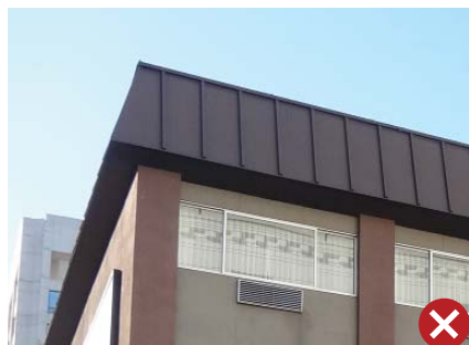
Inappropriate use of standing seam at roof.
