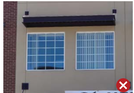
Inappropriate vinyl material.
