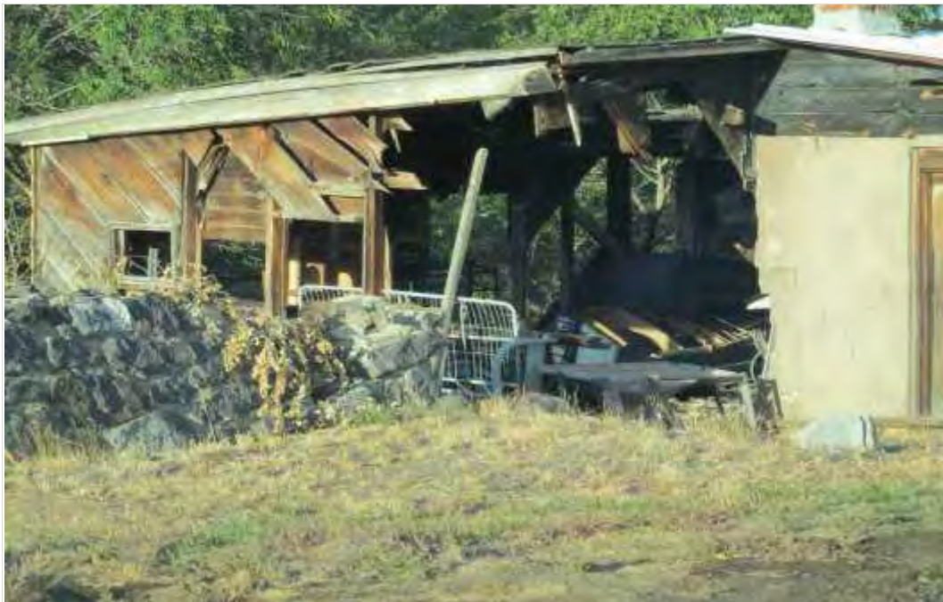
Abandoned/ Damaged Improvement Adjacent the Subject Lot
