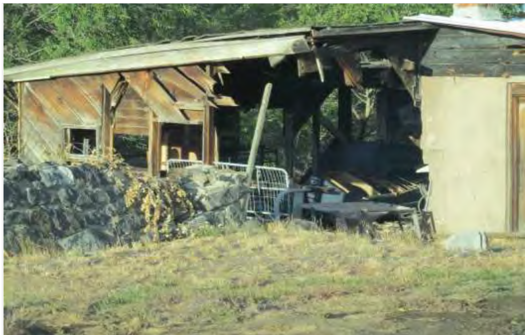
Abandoned/ Damaged Improvement Adjacent the Subject Lot
