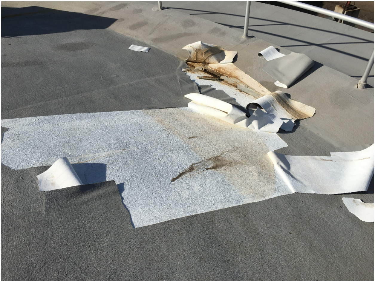
Photo 18: Non-adhered coating around blisters on digester cover exterior removed by hand
