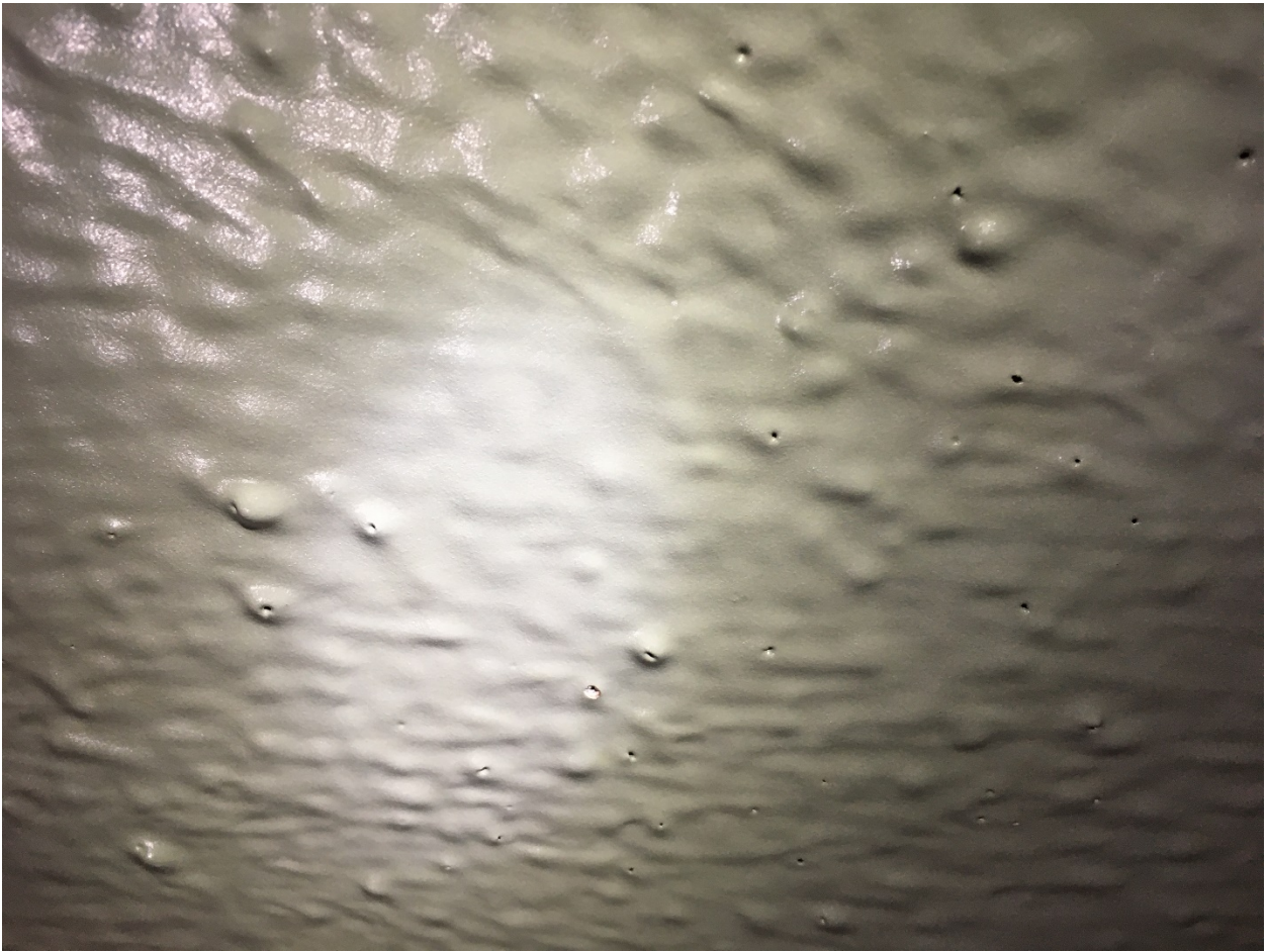
Photo 9: Closer view of digester cover interior coating pinholes
