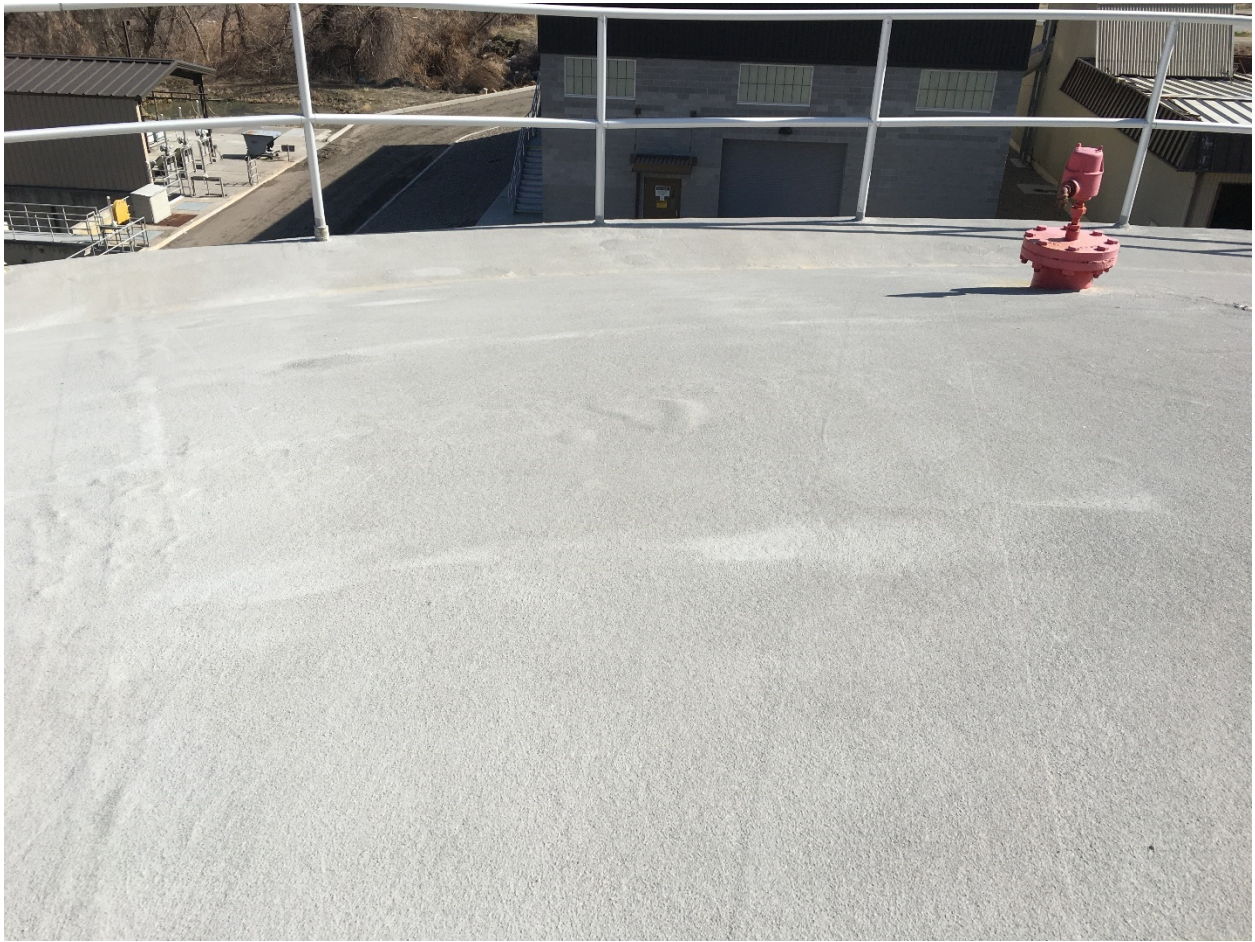
Photo 12: Overall view of digester cover exterior, showing coating blisters
