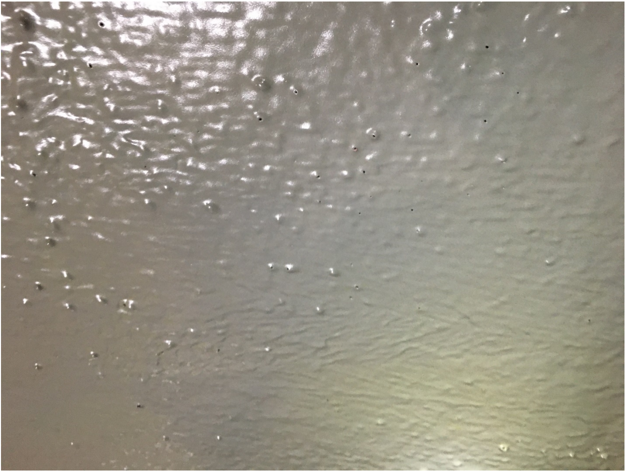
Photo 8: Close-up view of digester cover interior showing pinholes in coating
