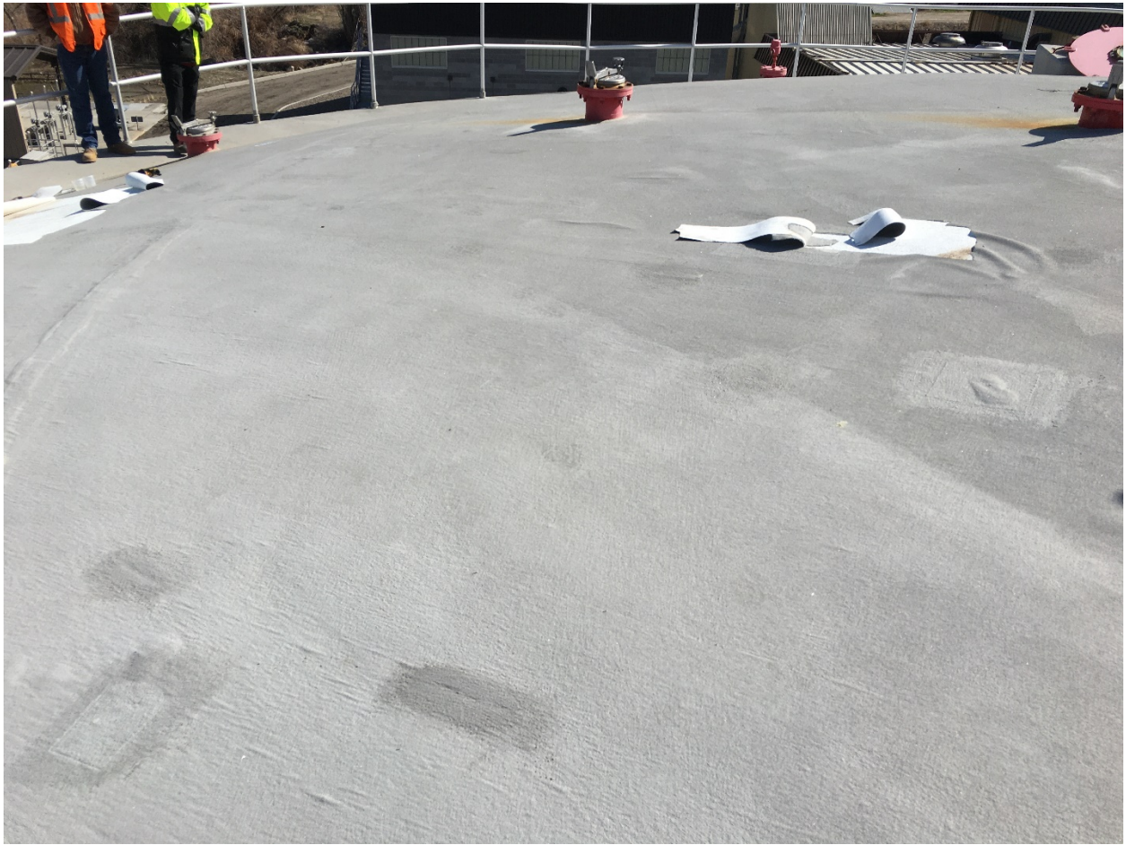
Photo 13: Overall view of digester cover exterior, showing coating blisters
