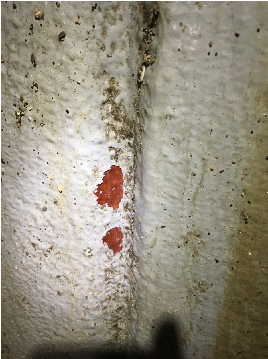
Photo 5: Top coat failure at interior joint of digester skirt, otherwise showing well adhered coating
