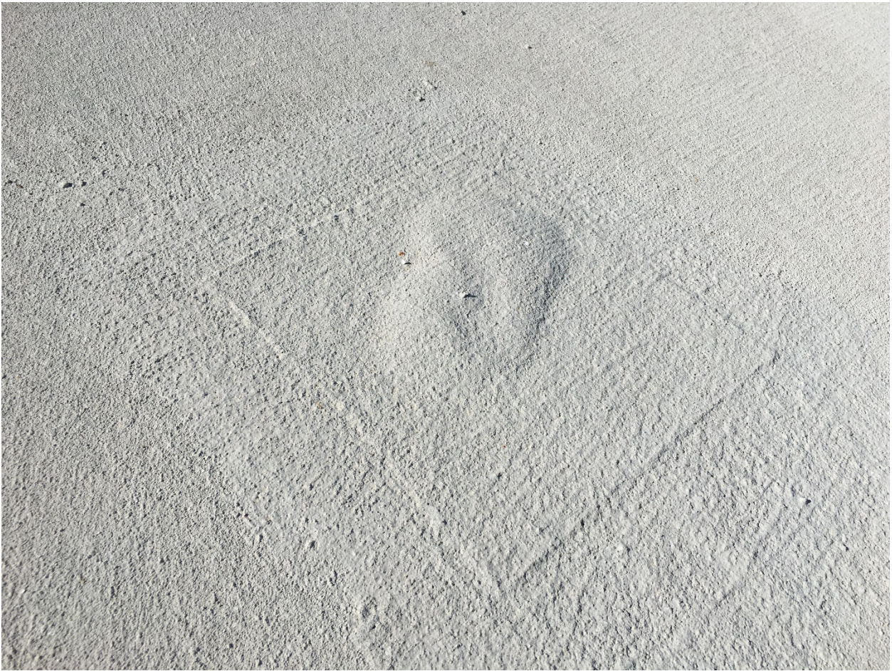
Photo 15: Coating blister at previous repair location on digester cover exterior
