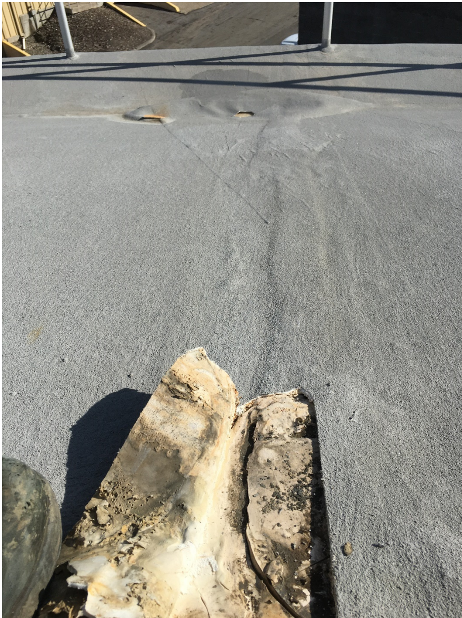
Photo 16: Coating blistering and joint grout damage on digester cover exterior
