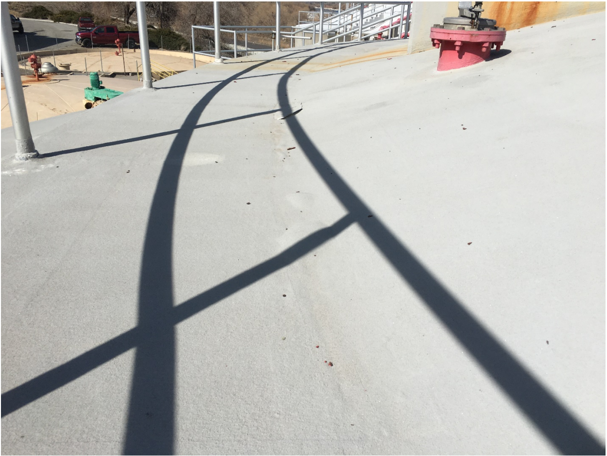
Photo 14: View of digester cover exterior dome perimeter, showing coating blisters
