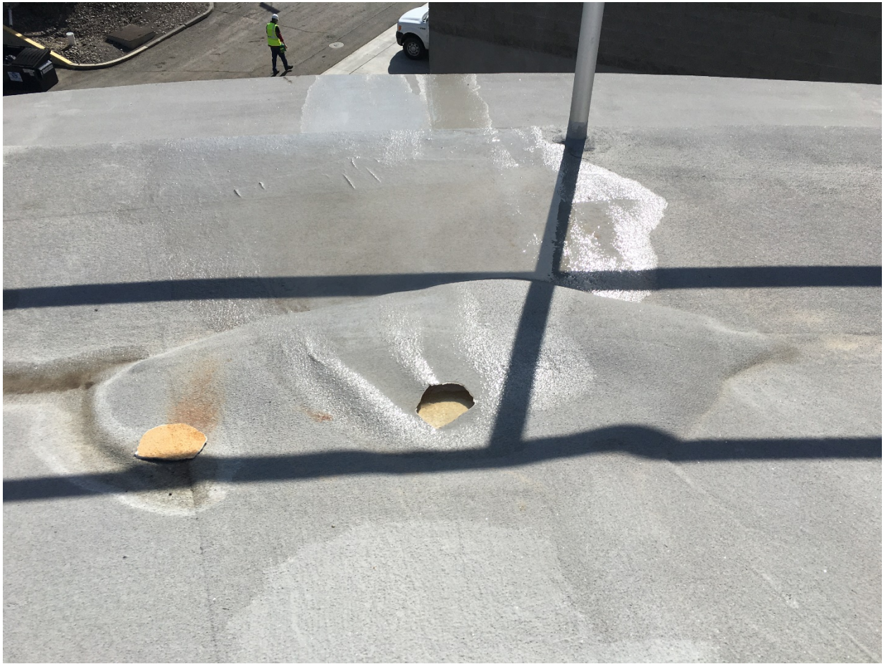
Photo 17: Digester cover exterior coating blister with accumulated water
