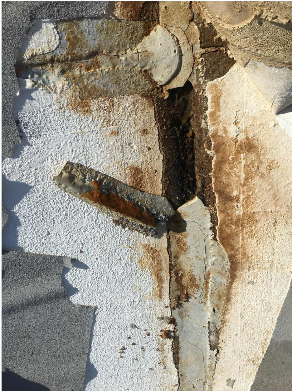
Photo 19: Damaged joint grout beneath blister along digester cover exterior dome perimeter
